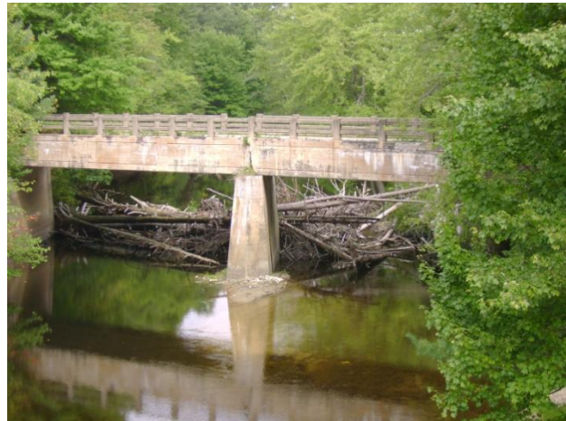
Photograph 9. Large debris dam on the Crooked River that was breached in 2007 and removed in 2008 (MDIFW Staff).
